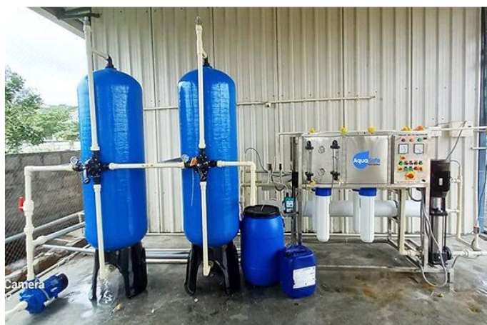
Installed 10 RO plants of 250 LPH at Gadag and Raichur for poor and underprivileged people
